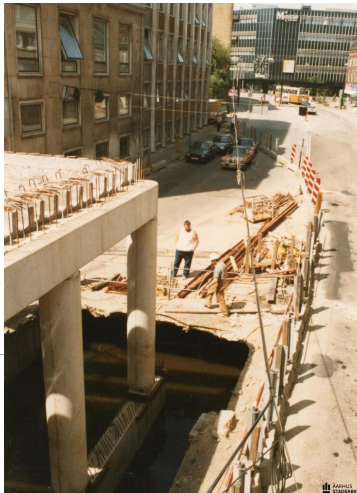
Constructing the new St. Clements Bridge with a look to The River Aarhus, 1984. https://www.aarhusarkivet.dk/records/000347545
