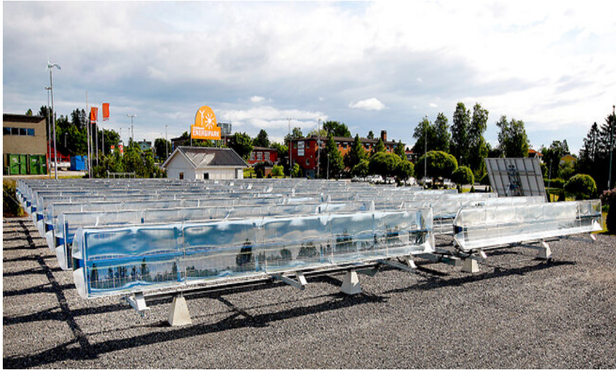
Photo high plain Solar Thermal Park – demonstration plant source: www. Processnet.se
